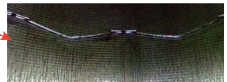
Oil filling hole area
