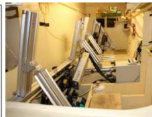
Figure 4: Measurement setup inside the steering gear compartment
